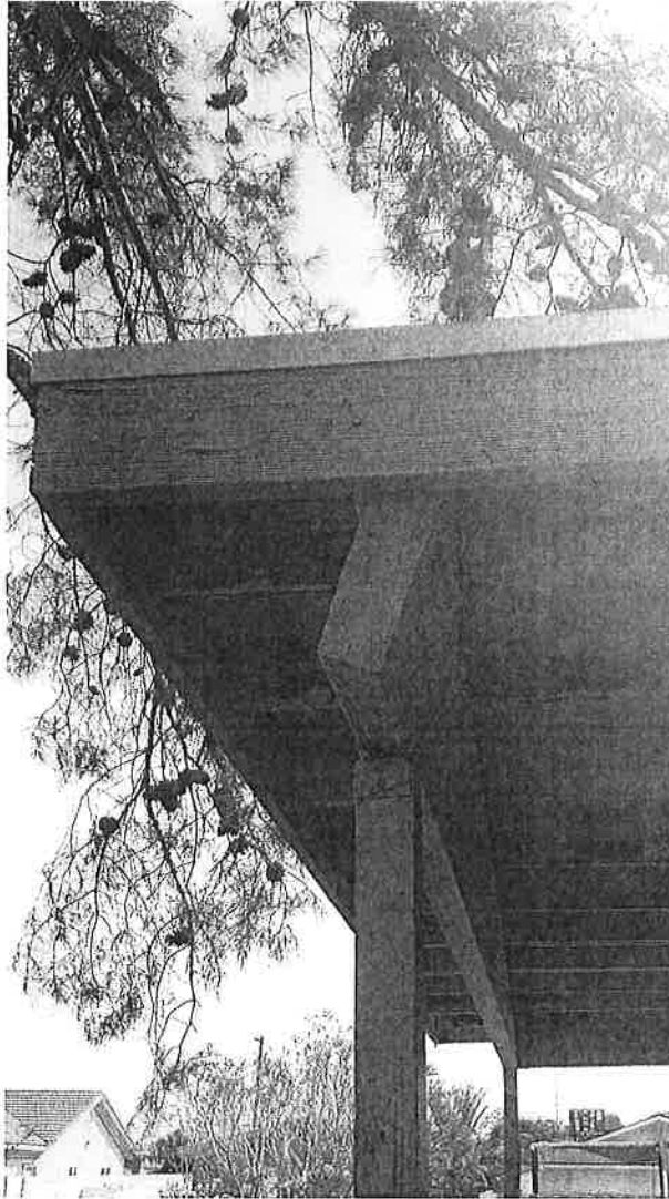
Photo 3 – Twist in Timber and Distorted Column Connection.
